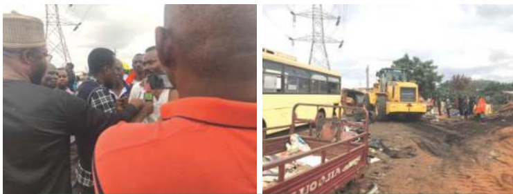
Demolition of illegal structures on VRA's natural Gas Pipeline Right of way
